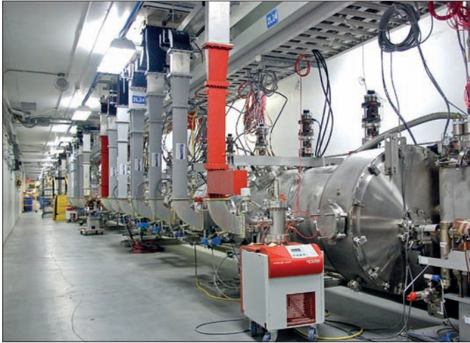
A cryomodule for the 12 GeV upgrade installed in the CEBAF accelerator tunnel.
