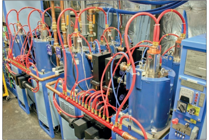
Eight new klystrons recently installed as part of the 12 GeV upgrade. A total of 80 new klystrons are required to provide the RF power for the complete upgrade.
